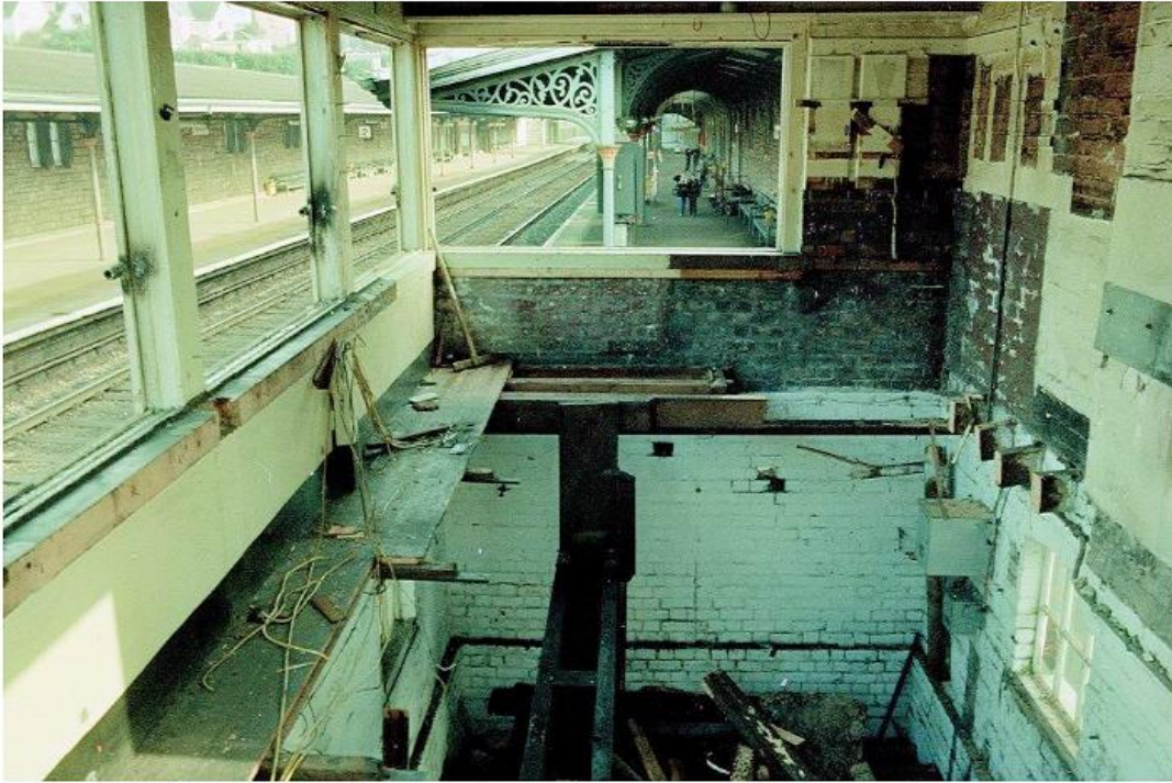
8. Inside Teignmouth box which was demolished that night. 14th Feb 1987 Copyright Paul Barlow
