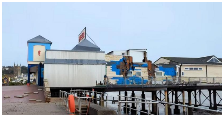
Storm damage Nov 2023.
