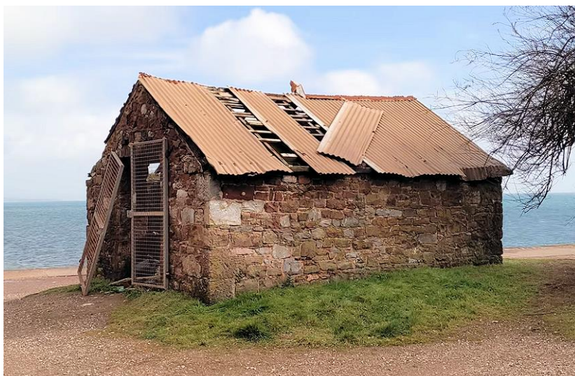
The sea wall gangs tool hut in later years. It is a protected building so will not be demolished.
